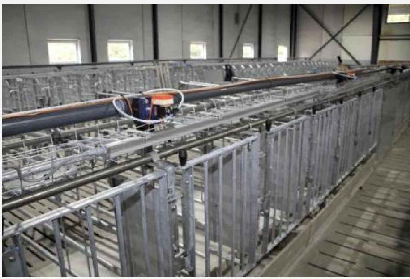
Here, another insight into how the led light runs parallel to the feed string, which can feed individually down to three or four lakes. Parts of the feed string are laid below floor level to provide so good view of the barn.
